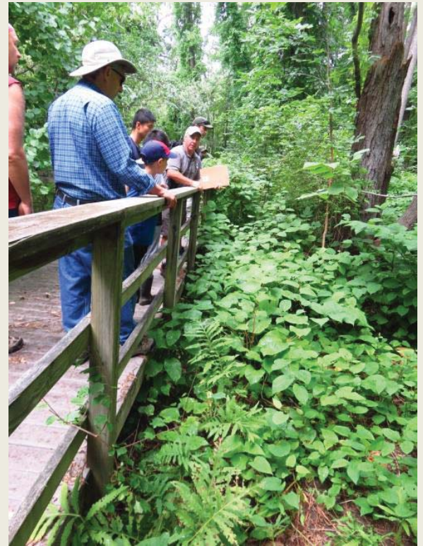
Footbridges need clearing and maintenance
