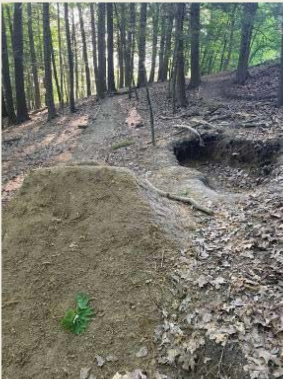
Digging and mounding of earth in riparian corridor can cause erosion and pollution of stream
