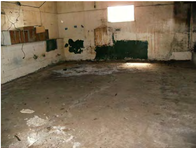
View of the dry feed weigh up room. Staining was observed on the floor and walls in this area.
