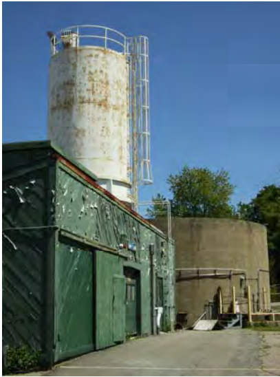
View of the wastewater pretreatment plant (lime silo and neutralization tank in background).
