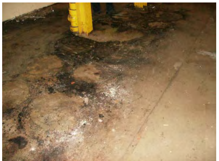
View of staining observed on the floor in the mixing room.
