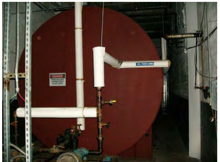
View of the 20,000-gallon No. 6 oil AST located adjacent to the boiler room.
