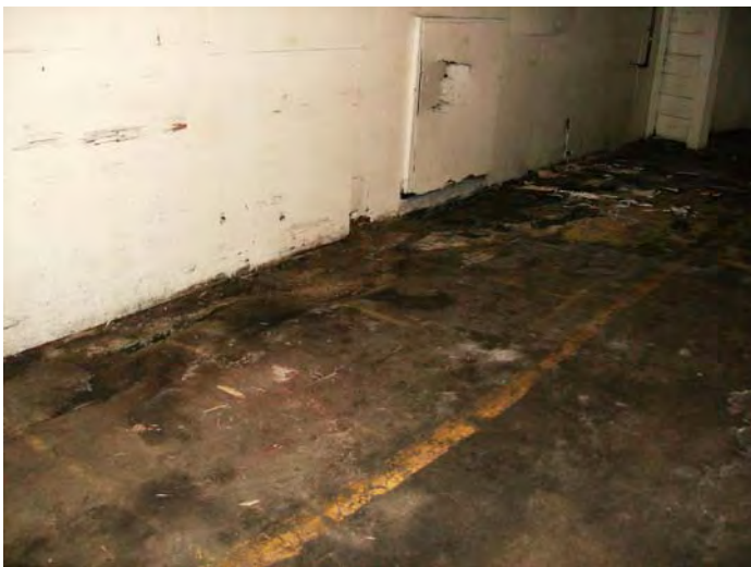
View of staining on the floor in the wet chemical storage area. The floor was observed to be in poor condition.
