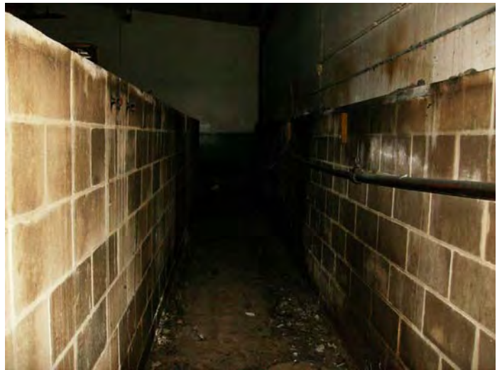
View of the location of a former conveyor where grease was heated with steam coils.
