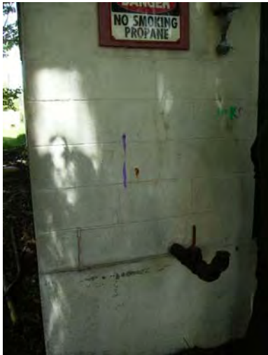
View of the fill pipe connected to a 3,000-gallon No. 2 fuel oil AST in the former Blue Sort Building (staining was observed on the fill pipe).
