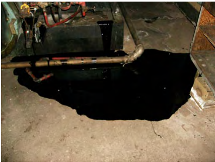
View of No. 6 oil on the floor in the boiler room.
